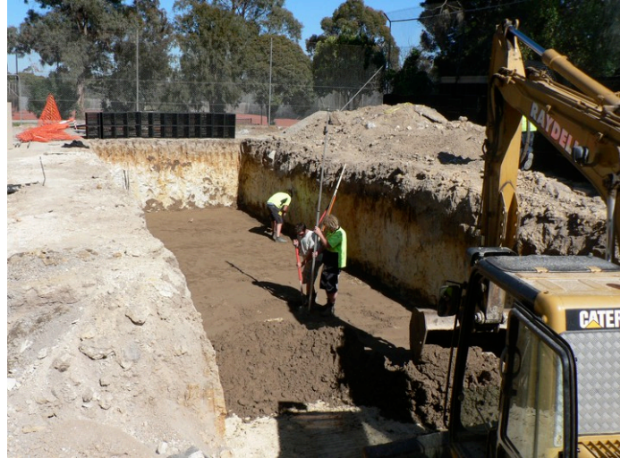
50,000 litre stormwater tank installation below the car park funded by a water authority grant at St Alfred's Church and used for cooling and irrigation
