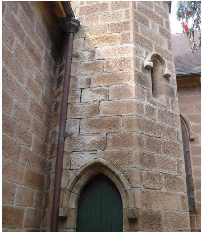
Costly stonework repair required after blocked rainhead has been overflowing.
